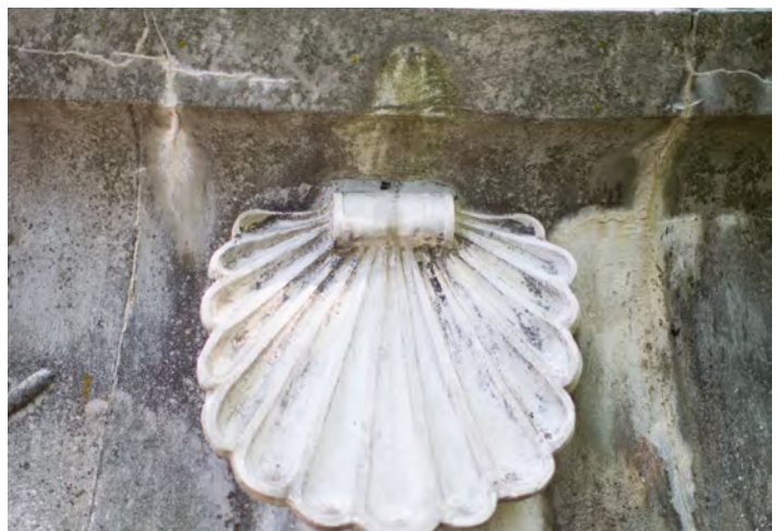
Figure 49: View of weep holes at shell, cracked limestone mineral deposits and trailing water
