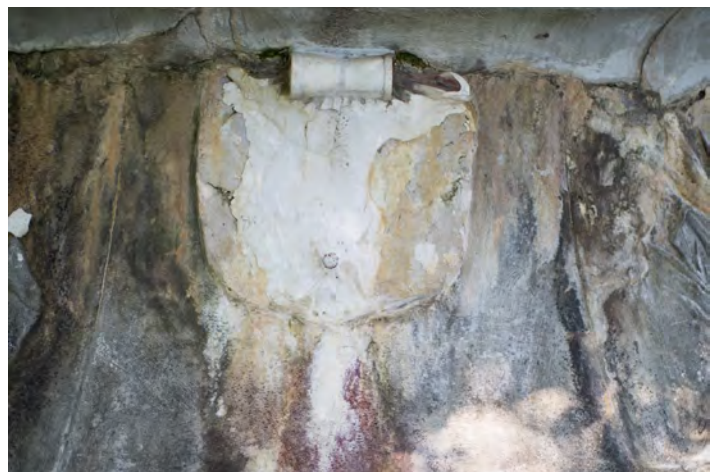
Figure 52: View of missing shell
