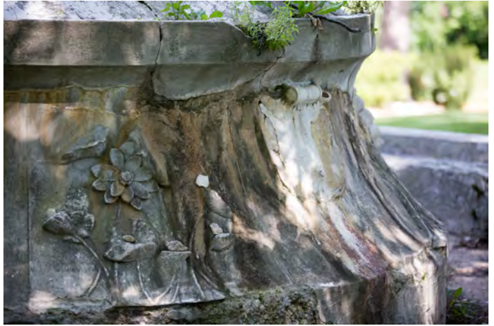
Figure 29: Excessive damage and improper repair with organic growth that is indicative of the level of disrepair
