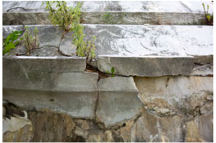
Figure 41: View of extreme damage to the limestone
