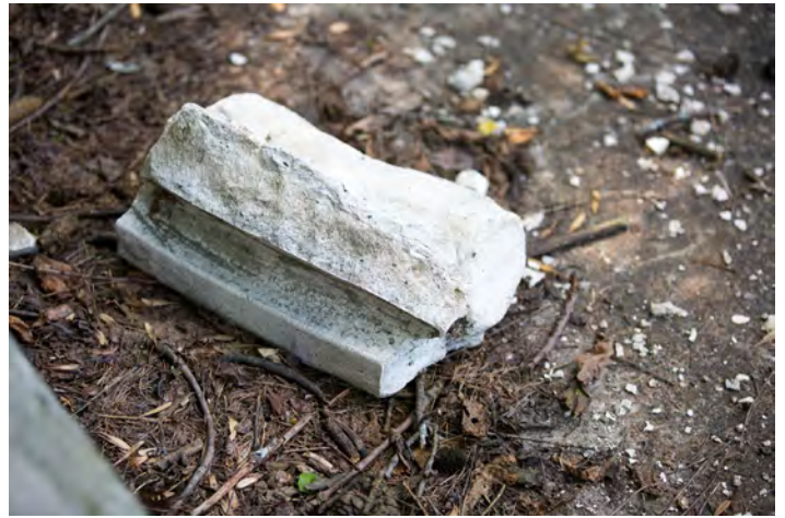
Figure 23: Broken piece on the site
