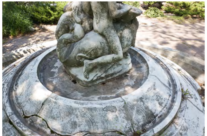
Figure 6: View of marble figures and upper view of pedestal and base - note damage to pedestal has been repaired and appears to have stabilized
