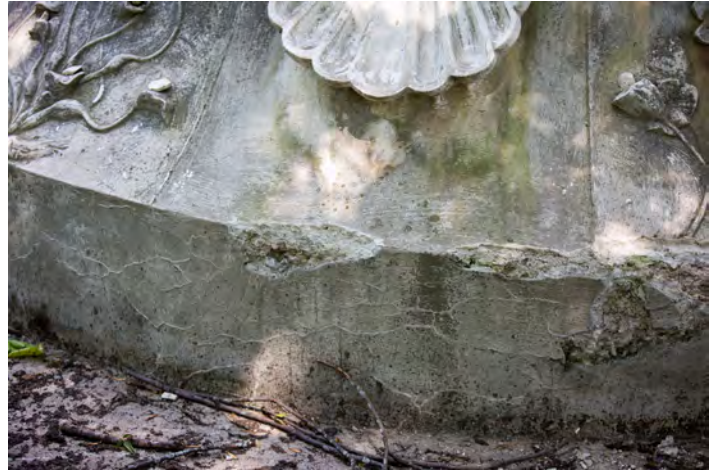
Figure 32: Degradation and mineral staining at trailing water
