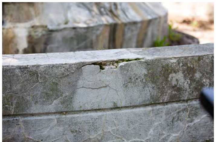
Figure 25: View of emerging damage at concrete at lower perimeter ring
