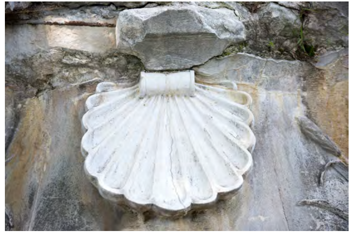
Figure 20: Shell motif condition amid limestone damage indicating restoration or replacement at some point in time
