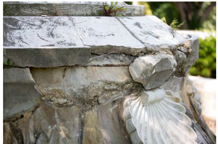
Figure 42: View of damage at tension ring
