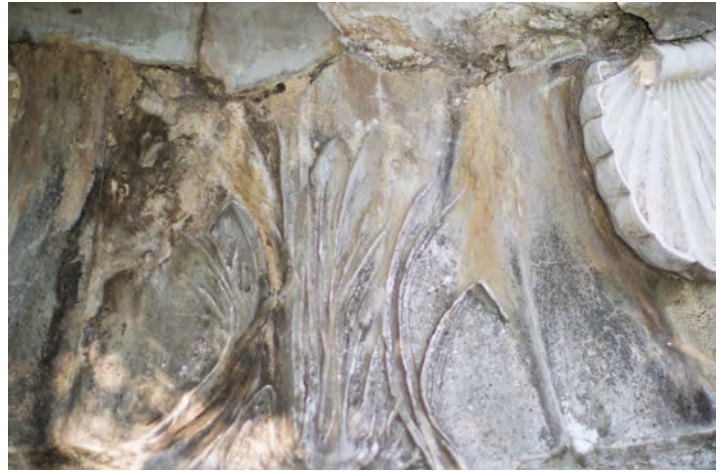
Figure 53: View of degraded material at cattail motif
