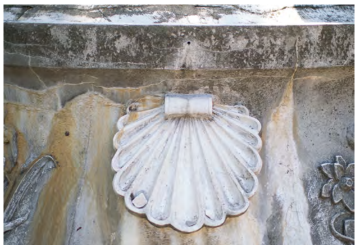
Figure 46: View of weep holes, cracked limestone mineral deposits and trailing water
