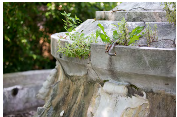
Figure 43: View of plant infestation and damage
