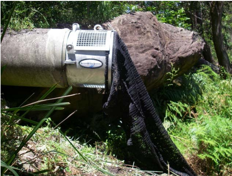
Figure 1. Example trash net to collect gross solids entrained in runoff.
